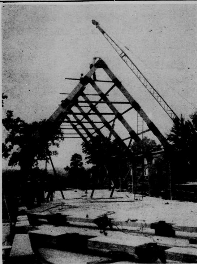
This photo shows workmen placing the huge arches for the sanctuary of the new Christian church here last week. At the time the photo was made, six of the nine arches were in place, with part of the remaining three to be seen in the foreground.
