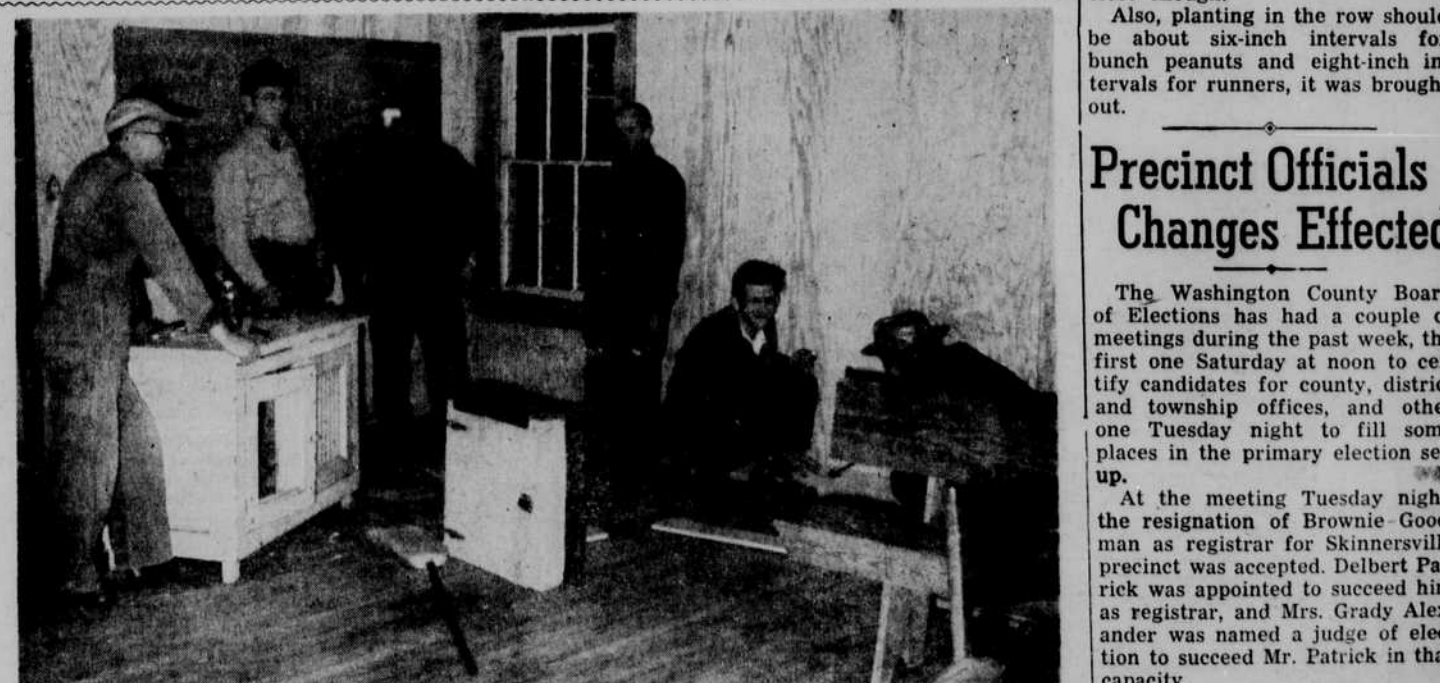
SCOUTERS: The Plymouth Boy Scout hut now boasts new wall and ceiling paneling, contributed by Atlas Plywood Corporation and installed in recent weeks by members of the troop committee and parents and family. Left to right, the above group was caught as they finished up the work there last Thursday night. Left to right, they are: Robert Howell, chairman of the troop committee; Joseph Mizelle, Lyman Mayo, C. A. Walker, William B. Blackburn and Borden Kornegay.—Staff photo.
