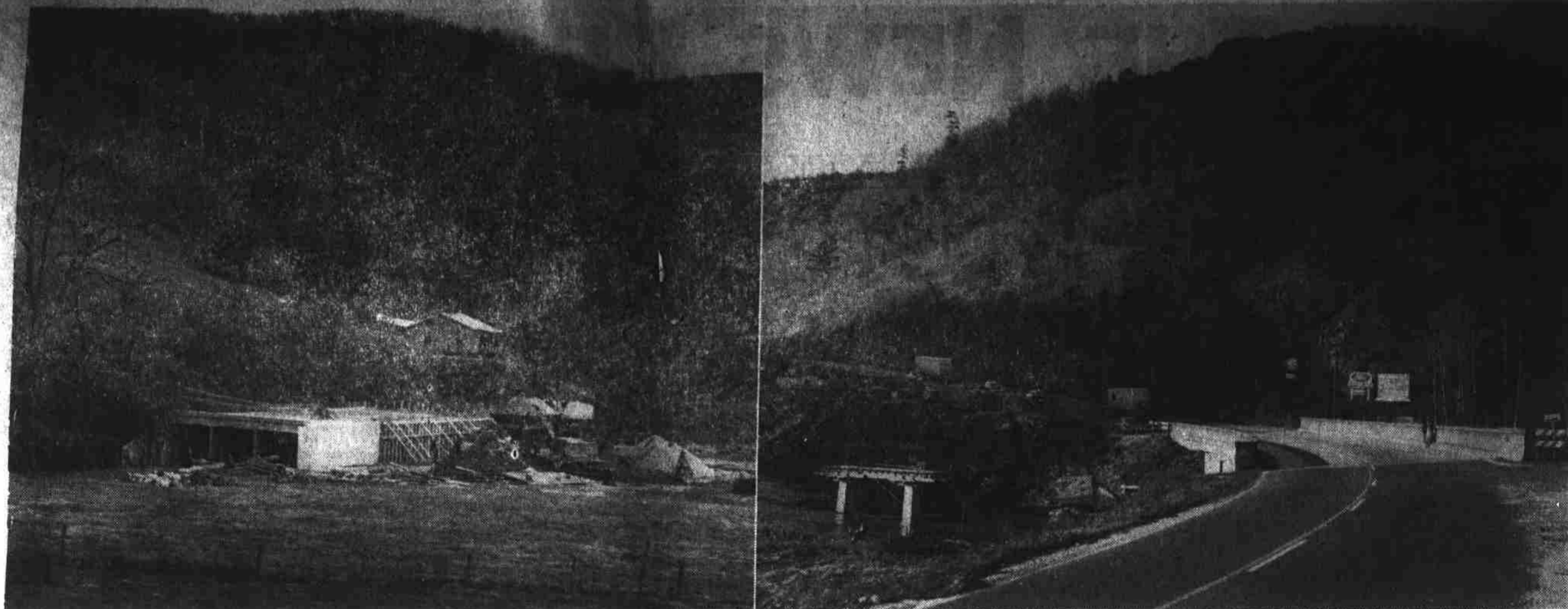
HIGHWAY STRUCTURES are now being built for the new bypass which will carry U. S. 25-70 around Marshall. At left, a bridge is under construction across Walnut Creek half a mile from the point at which the north end of the bypass will link with
