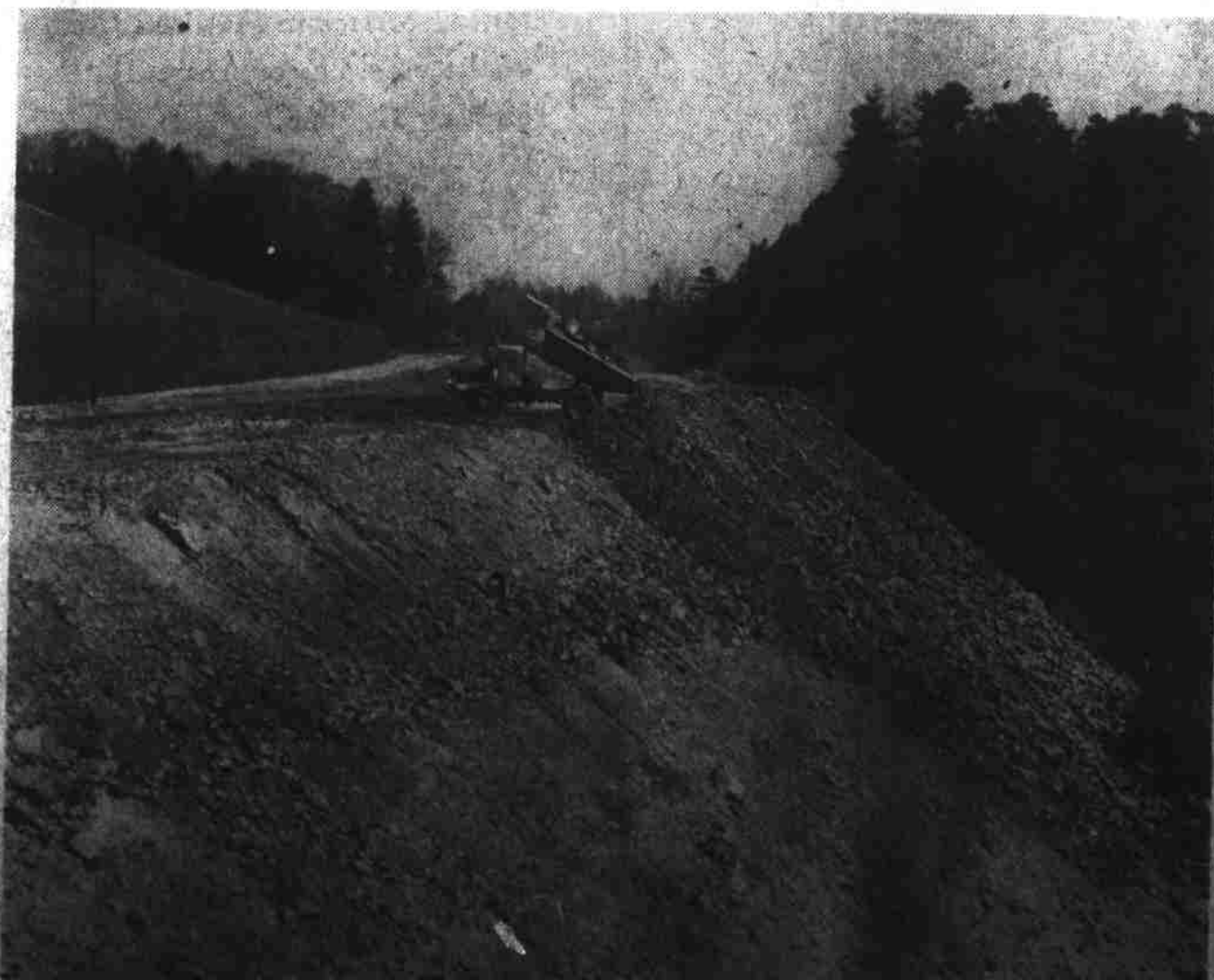
Pictured above is a portion of the Marshall Bypass which is rapidly being constructed. Officials state that the new two-lane highway will be ready for use this fall. Two bridges are also being built
