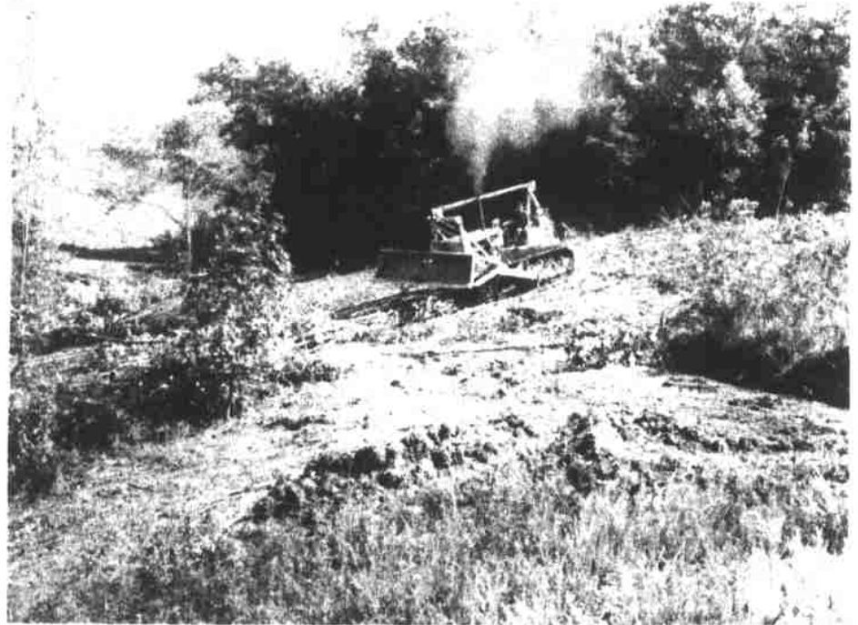
THE FIRST VISIBLE evidence of construction of the Madison County High School was shown Monday morning adjacent to the Marshall By-Pass, site of the school. The clearing of the undergrowth is essential for preparation of core-drilling equipment that the board of education expects to be moved in within the next few weeks. The citizens of Madison County voted overwhelmingly last May to approve a Bond Referendum of $950,000 to consolidate the five existing high schools into a single comprehensive high school.
