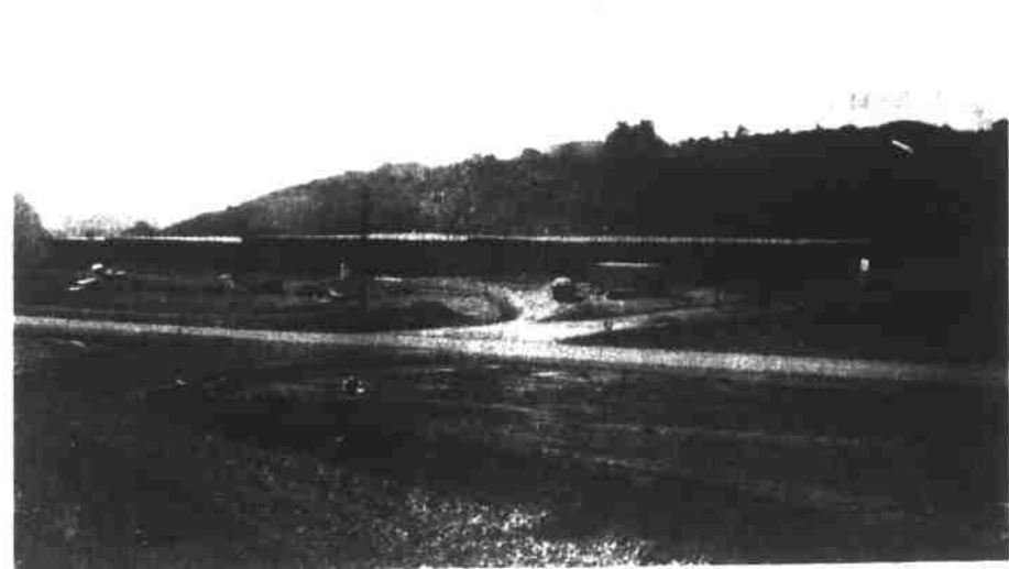
PICTURED ABOVE is the future shopping center located on the Marshall by-pass. Recently added to the progress of the project is the roof. Picture taken from the approach to the consolidated high school, now under construction.
