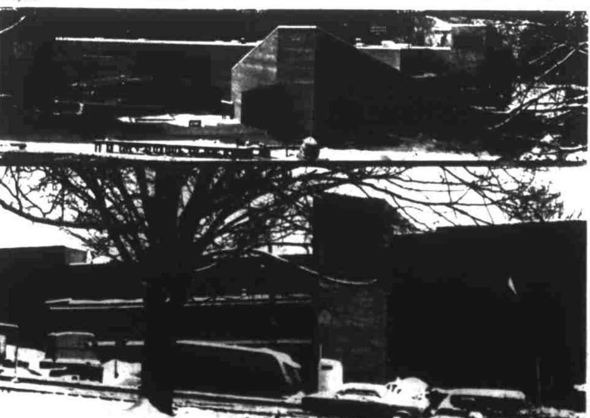
THE TWO NEW BUILDINGS under construction on Mars Hill College campus—the College Union (top) and Cornwell Hall—were more than three-fourths completed when the first heavy snow of the winter fell in early January. The contractors have promised full completion by early spring, and college officials are planning "open house" activities in both structures during commencement weekend, May 19-20. The College Union, a $1.1 million project of Engineers-Constructors, Inc. of Knoxville, wedges interestingly between the science building (left), the cafeteria and the football stadium. Cornwell Hall, a combination of classrooms and faculty offices, occupies a strategic position facing the little circle at the center of the campus. A $457,800 project of Buncombe Construction Co., it is named for trustee George T. Cornwell '27 of Morganton.
