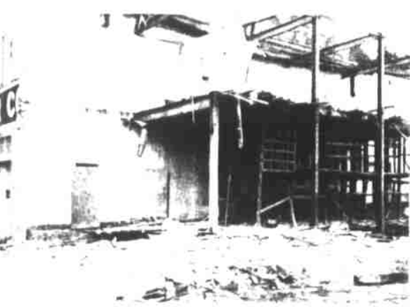
THE ABOVE picture looks like an earthquake has just demolished the back of Coal, Feed & Lumber Company building on Upper Bridge Street here. However, repair is underway on the building which was struck early Saturday morning, Jan. 22, 1972, by a Southern Railway freight train which derailed with 17 freight cars involved. Damage will also necessitate extensive repairing to the front of the large building.
