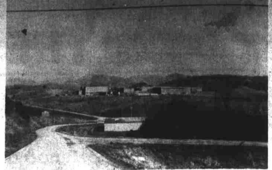
CONSTRUCTION CONTINUES on the Madison County High School on the Marshall By-Pass. The facility, when completed, will be one of the finest in Western North Carolina. The above picture was taken Sunday afternoon from the road leading to Mato Packing Company from the Marshall By-Pass.
