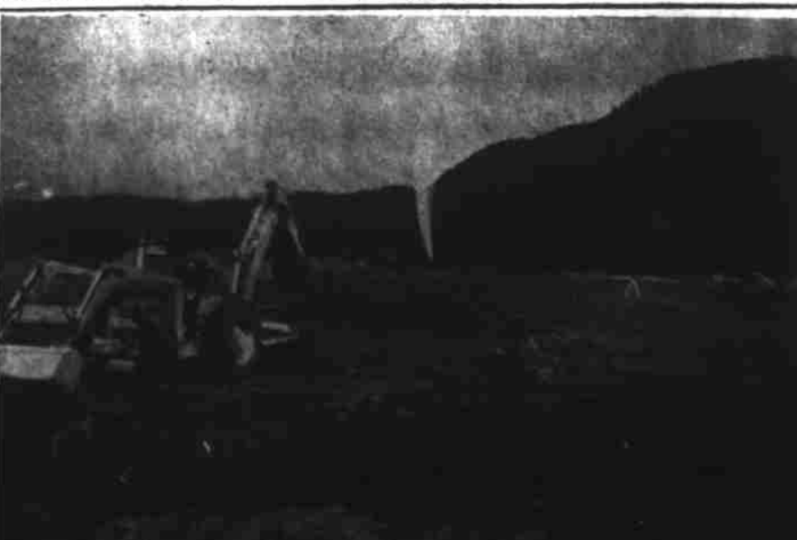
CORE DIGGING and pouring footing for the construction of the Hot Springs industrial building is now underway. When completed the building will contain 38,000 square feet and is located on the Barber Foster property.
