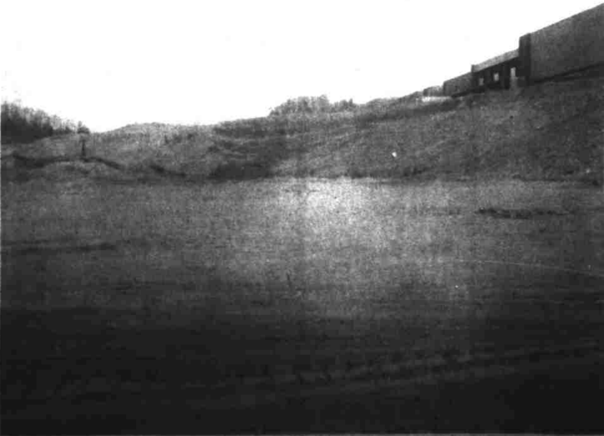
FUTURE FOOTBALL FIELD at Madison High School is being constructed and it is hoped that the stadium will be ready for use this Fall. A portion of the high school is pictured at right top.
