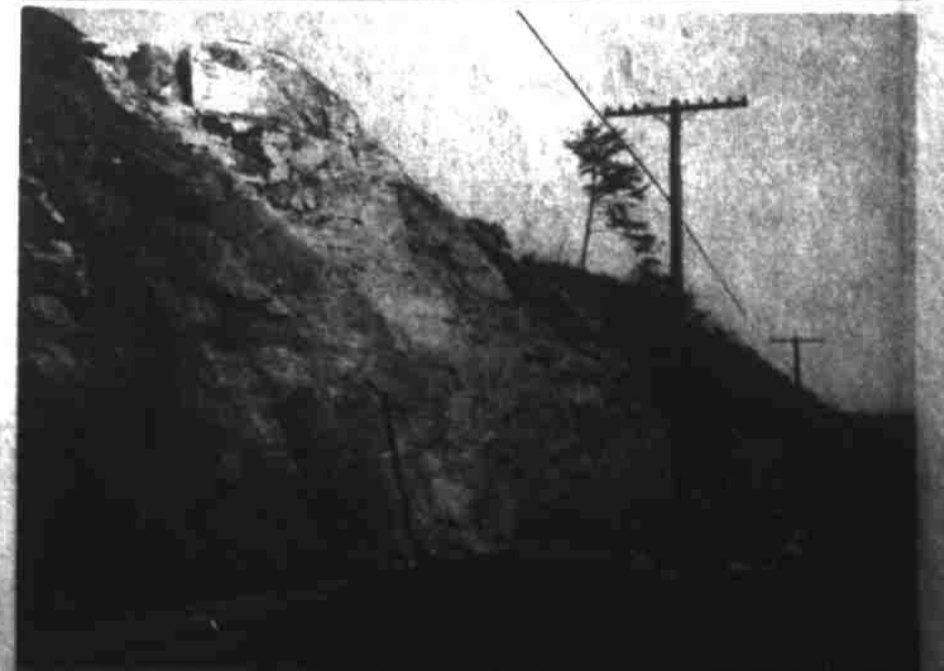
DANGEROUS OVERHANGING ROCKS between Marshall and the Ivy Bridge on US 25-70 Business are pictured above. Motorists have been delayed via the Marshall by-pass for weeks. Landslides, large cracks, and loose boulders have been caused by blasting for stonehills material for highway and railway maintenance, as well as continuous wet weather.
