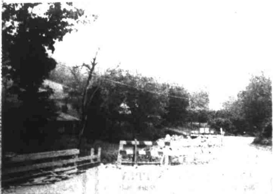
NC 213 CONSTRUCTION between Marshall and Mars Hill is continuing. Short detours, such as shown above, are commonplace. The above picture was taken Saturday near residence of Mr. and Mrs. Hilliard Teague on Hayes Run. The long detour near Mars Hill has been removed, much to the delight of everyone. The completion date for the relocated and improved highway is set for 1977.
