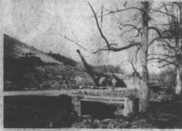
CONSTRUCTION ON NC 213 continues between Marshall and Mars Hill. Similar scenes as above are commonplace as heavy machinery and workmen are changing the appearance of the highway. Above picture taken in front of the residence of Mrs. Ethel Sprinkle on Hayes Run.
