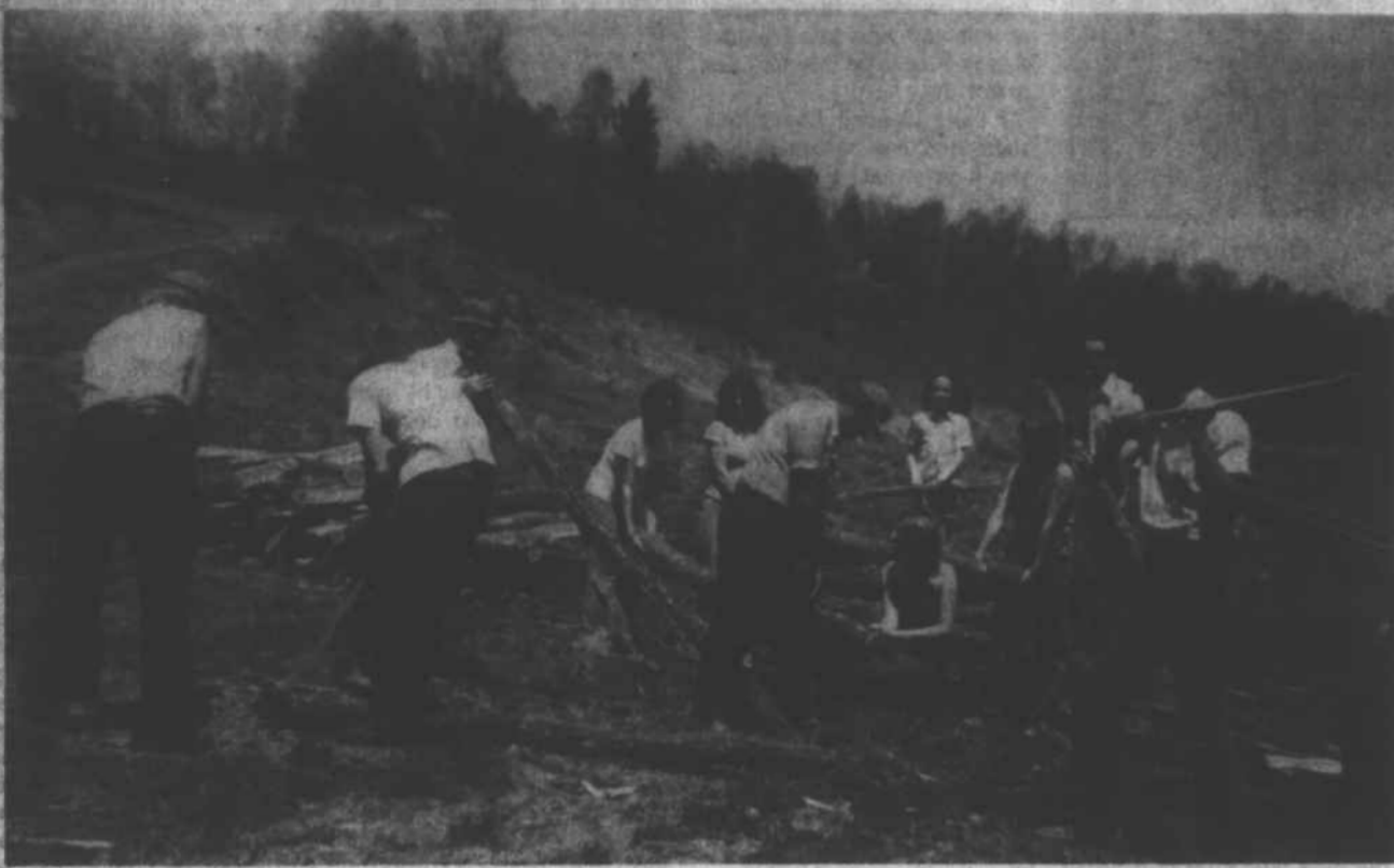
THE LITTLE Ivy Baptist Church youth group is presently engaged in building a recreational area for their church. The property was donated by J. C. Young, and is
