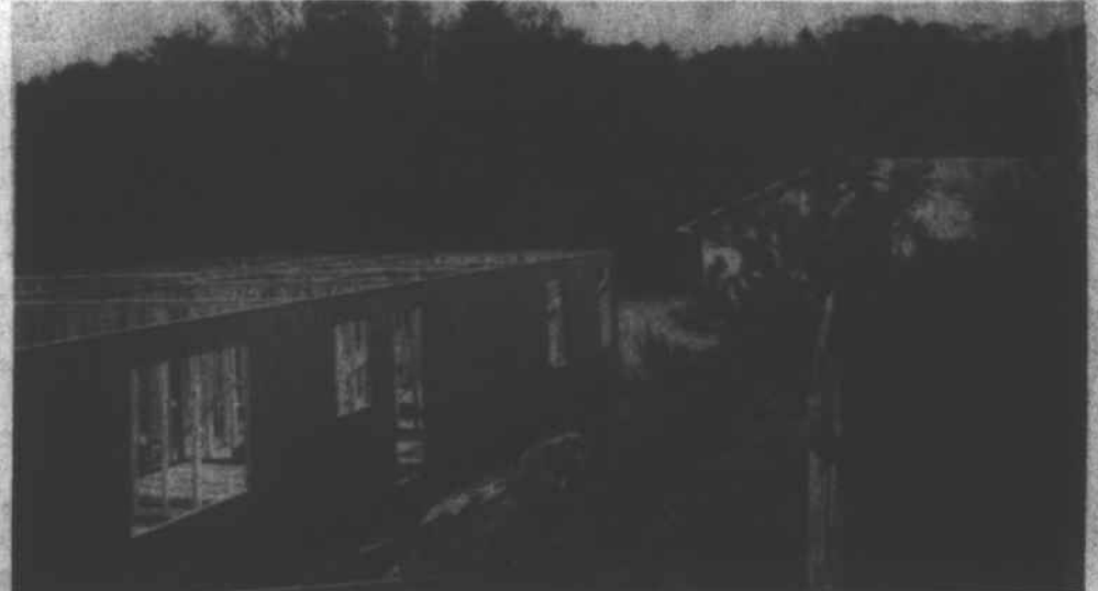
TWO PARTIALLY constructed rest homes (above) located in the Rector's Corner area near Marshall, are expected to be open by Jan. 1. (Photo By Jim Story)
