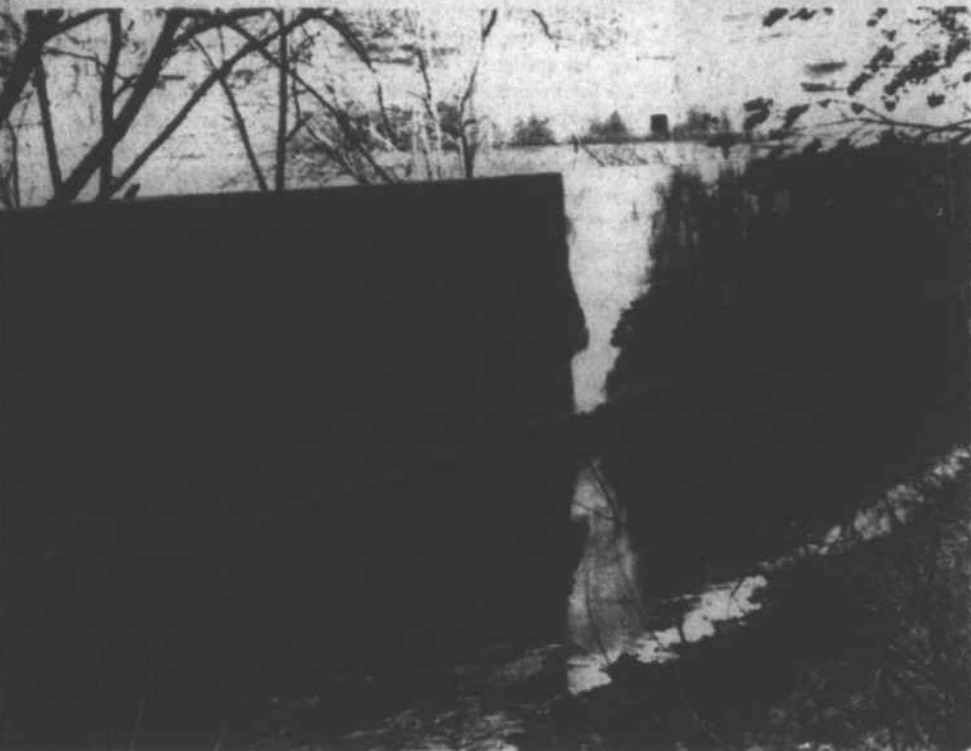
THE EXISTING SLUICEWAY at the old Capitola Dam site, built around 1910, will play an important part in the hydroelectric generating facility proposed by French Broad Electric Member-
