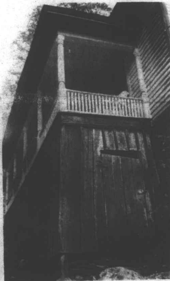
BEFORE AND AFTER—Work has begun on Mrs. Ella Baker's house as part of the Town of Marshall's Community Development project. The photo at right shows some of the preliminary work being done to the exterior
