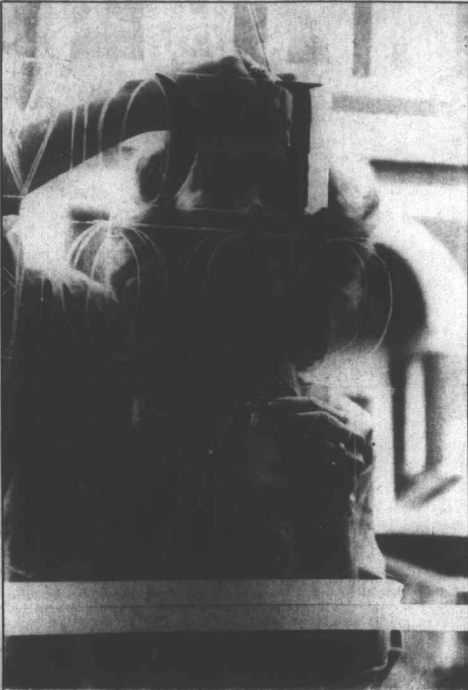
LADY SIGN PAINTER — Maggie Woods was busy painting a "Home Cooked Meals" sign on the window at Roberts Pharmacy in Marshall Thursday. The drug store is undergoing renovations to recreate an atmosphere of the "old timey" drug stores of
