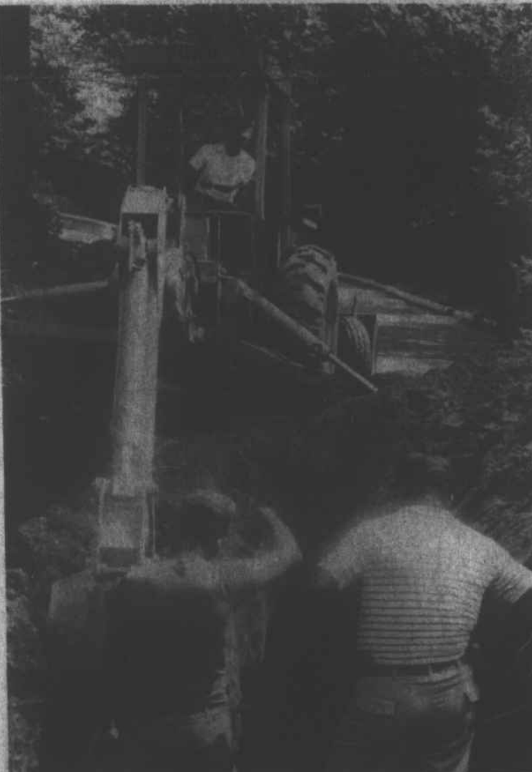
WORK ON THE MARS HILL SEWER PROJECT CONTINUED THIS WEEK. In photo above, Manuel Briscoe, right, oversees ditch digging near Mars Hill Elementary School.
