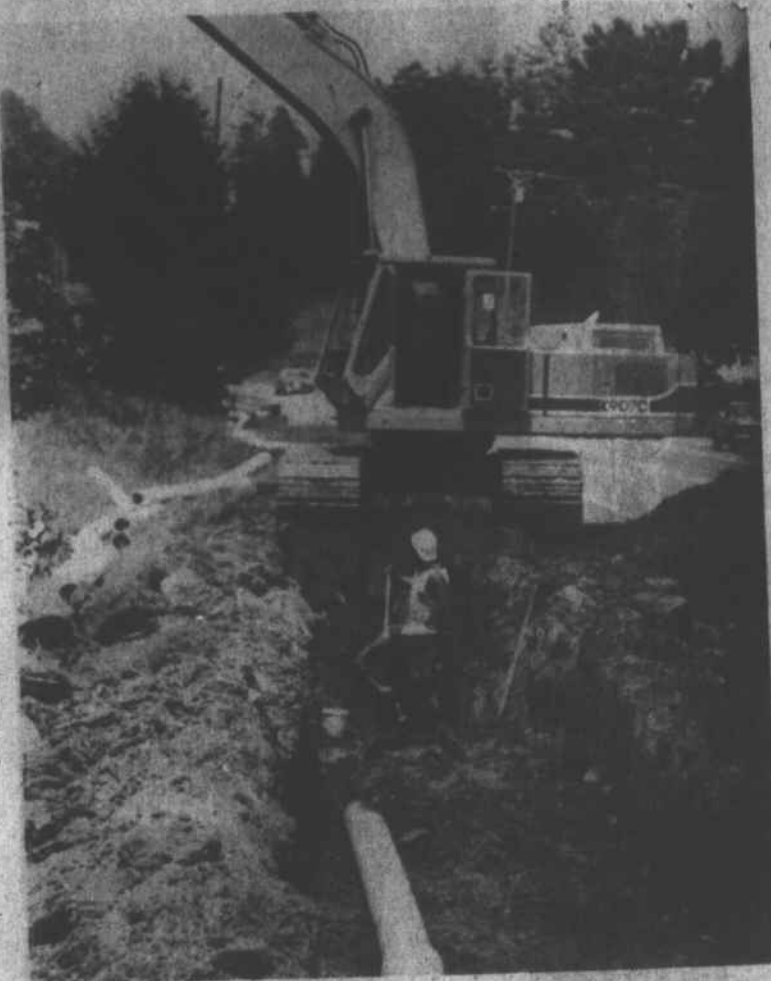
WORKMEN INSTALL SEWER LINE on Long Branch Rd. in Mars Hill on Monday. Work on the project is expected to continue on Hwy. 213 for several weeks.
