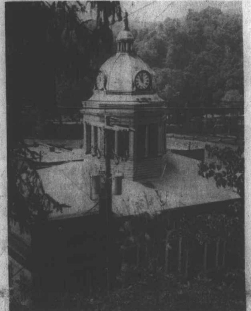
The dome of the Madison County Court House may have to be removed because of damage caused to the building's roof.
