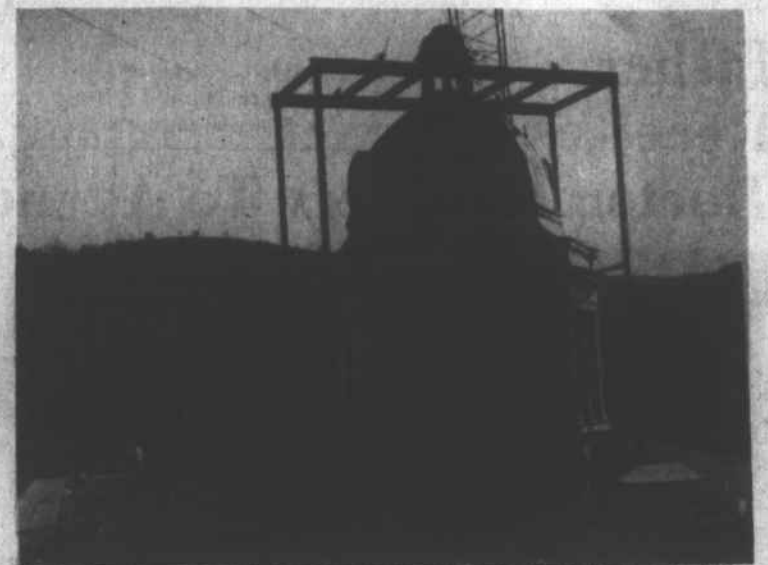
CUPOLA OF THE MADISON COUNTY COURT HOUSE was removed by workers on Saturday afternoon. Several hundred spectators gathered to watch the dome removal. More pictures on Page 5.
