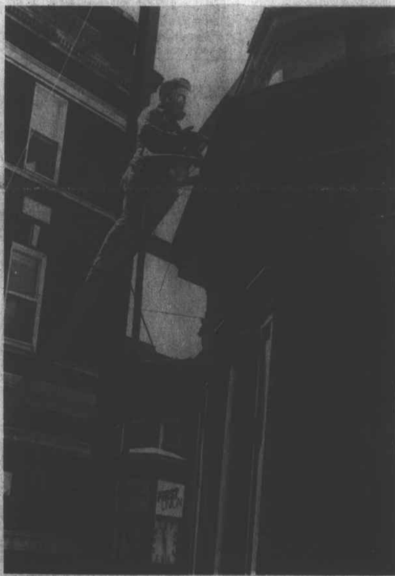
WORKMAN BLASTS OLD PAINT FROM county courthouse cupola. Restoration of the landmark continues as work on the courtroom is completed.
