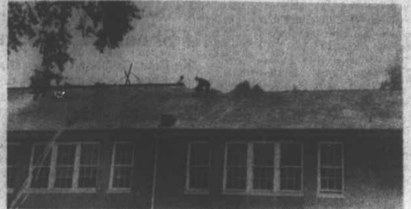
WORKERS REPLACE 59-YEAR OLD ROOF on Marshall Elementary School last week. Passage of additional half-cent sales tax will make other improvements to county schools possible.
