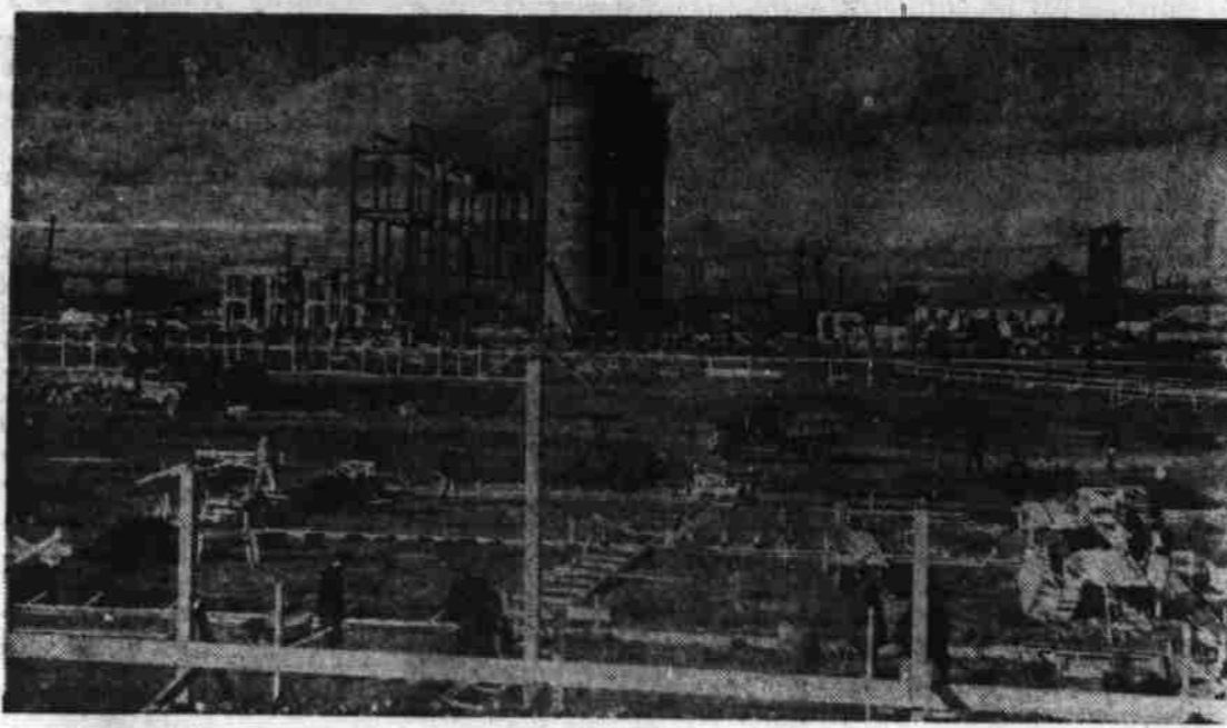
Just last summer this site was a cornfield and tobacco patch, which gives you an idea of how fast the government is working to overcome one of the defense bottlenecks. These buildings, rapidly nearing completion at Charleston, Ind., will form a tremendous powder plant for the army. (Central Press)
