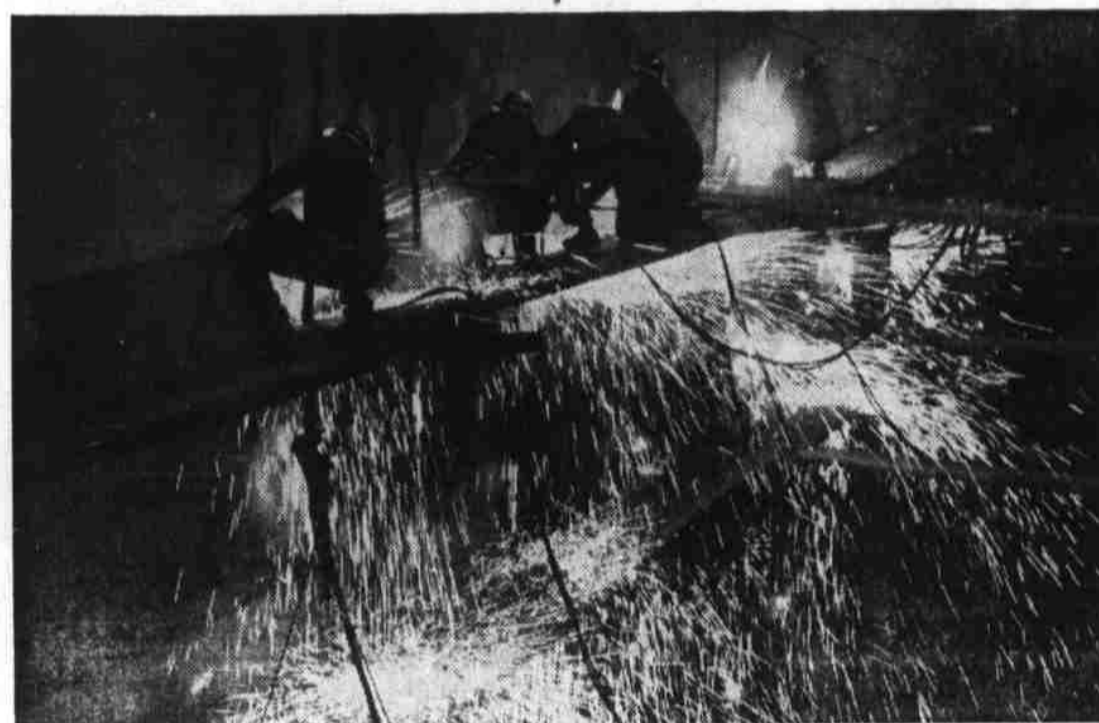
Along with sailors and merchant marine seamen, shipyard repairmen are doing their best to keep 'em sailing. This unique photo was made in the Todd shipyards in Brooklyn, N. Y., as a crew of welders use acetylene torches to repair a giant vessel in one of the drydocks. The men are removing bent plates from the side of the ship. (Central Press)
