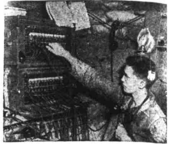
Telephone Switchboard in Dugout in New Guinea —U. S. Army Signal Corps Photo
