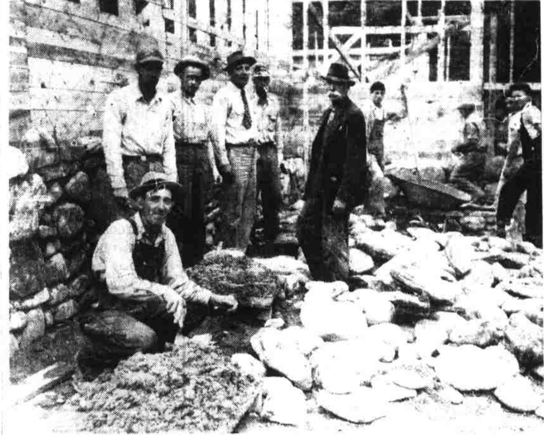
Shown here are a group of workmen putting up the rock walls on the $10,000 Rocky Branch Baptist church on Allen's Creek. Much of the labor is being contributed, and present plans are to complete the 40 by 62 foot building within the next forty days. Shown left to right, Jake Davis, T. R. Kirkpatrick, Fred Smith, Harry Hembree, Pless Kirkpatrick, Will Jordan, Leonard Smith, May Davis, Tommy Kirkpatrick and Guy Davis. Newton Davis, in charge of construction, and Abe Davis, are not shown in the picture. (A Mountaineer Photograph by Wallace Marley.)
