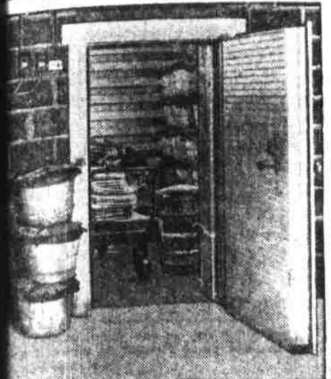
A typical walk-in cooler, with electrical equipment located to the left of the door.
