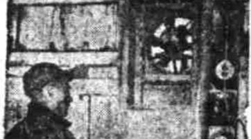
OUTTAKE FAN —installed in sidewall near ceiling with duct extending into within 20 inches of floor. Cover at top can be removed for summer ventilation and for servicing of fan.
