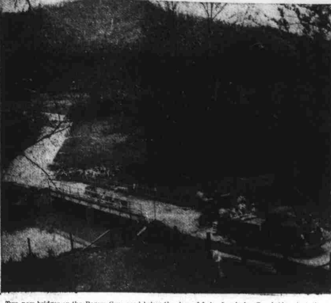
Two new bridges on the Rogers Cove road below the dam of Lake Junaluska. One bridge, just above the one shown here, has been completed, and this one, across the main stream of Richland Creek, is well underway. The new bridges will be wider, and the road straightened. (Staff Photo).
