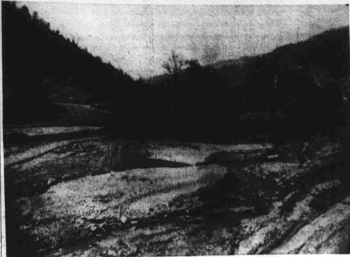
Heavy dirt moving machinery working like beavers were moving tons and tons of earth for the new dam at Daniel Boone Boy Scout Camp on Pigeon River. The dam was damaged by floods several years ago, and last spring a campaign was inaugurated to raise money for a new dam. This staff picture was made from the diving stand, looking towards the lake-side of the dam. The stream can be seen at the bottom of the picture. Several shovels, and a fleet of trucks and bulldozers are engaged on the project. (Staff Photo)
