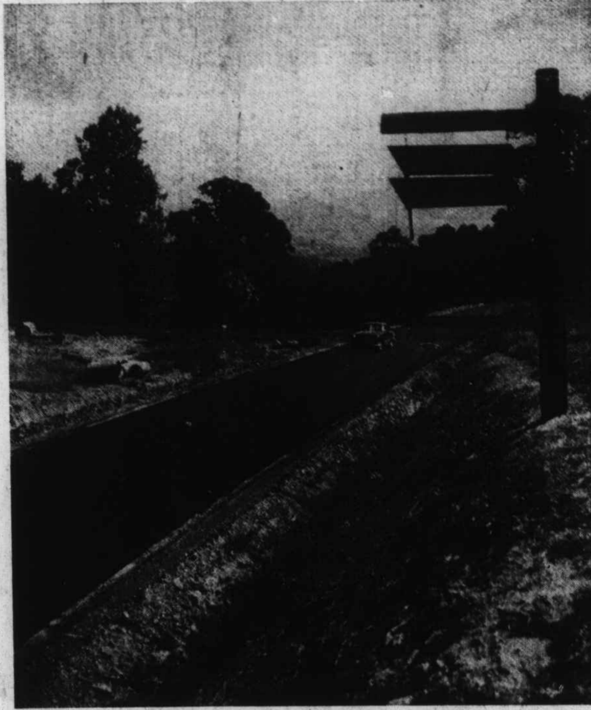
This week the hard surfacing of the new mile and a half stretch on Highway 276 was completed and the entire highway is now open to traffic. The new section takes out many of the dangerous curves of the old road and offers motorists a beautiful scenic ride through Pigeon Gap. (Mountaineer Photo.)
