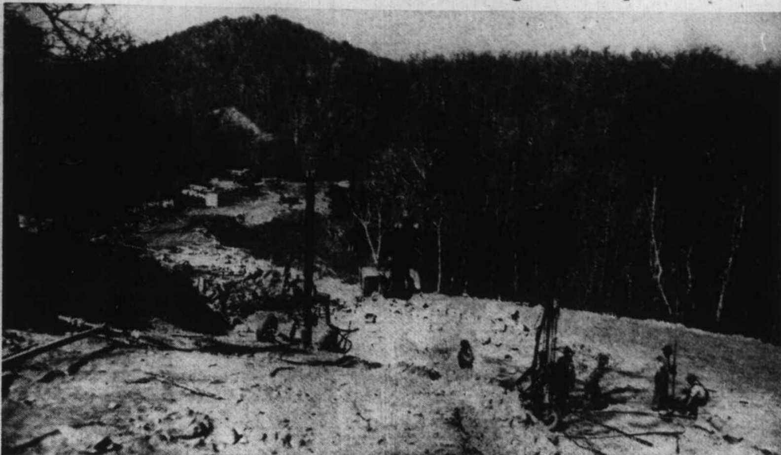
On March 1 Clement Bros. Construction Company of Lenoir started work on a four-mile section of the Parkway between Wagon Road Gap and Beech Gap. When open to the public, possibly a year from this spring, motorists will be able to drive the 12 miles between the two Gaps. The stretch now under construction will join at the Beech Gap end about 1 1/2 miles east of the tunnel at Devil's Courthouse. The crew is now making its first fill and a right-of-way about a mile long has been cut through the wood. The contract calls for the section to be completed in 500 working days at $400,000.
