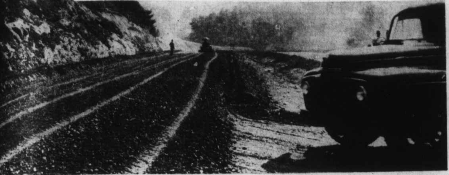
GRAVEL has been spread over the new four-lane highway from Canton to Lake Junaluska. This photograph was made by Mountaineer, as gravel trucks were nearing the end of the job at the intersection near the Lake. Several other coats of
