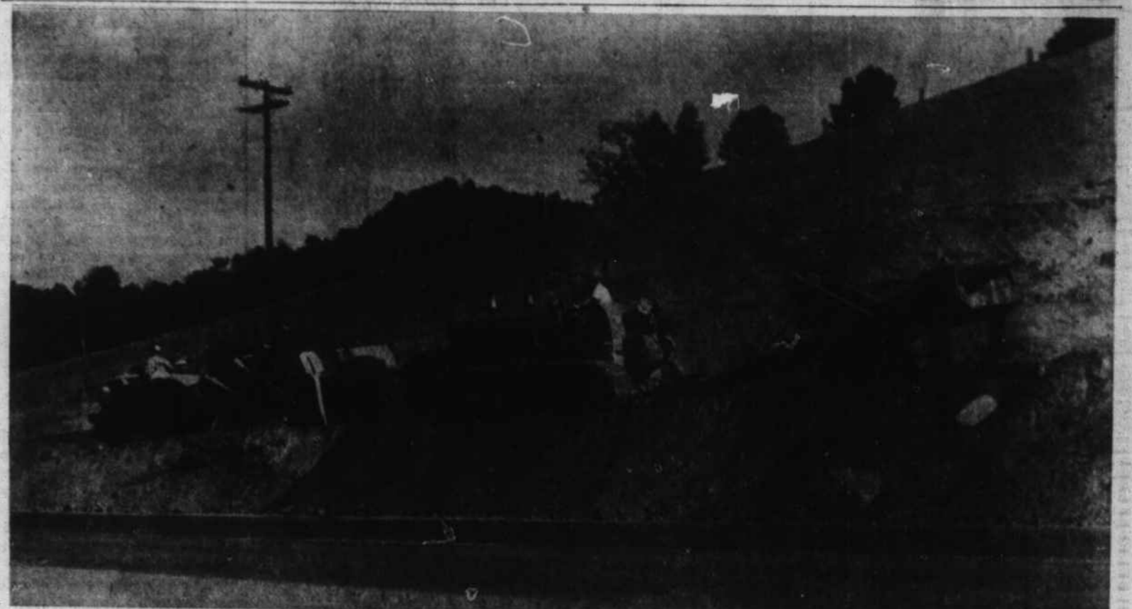
HEAVY MACHINERY is rapidly cutting into the hillside at Lake Junaluska at the intersection of Route 19 and 19-A as workmen of the H. R. Stewart Co. continue grading of the new four-lane
