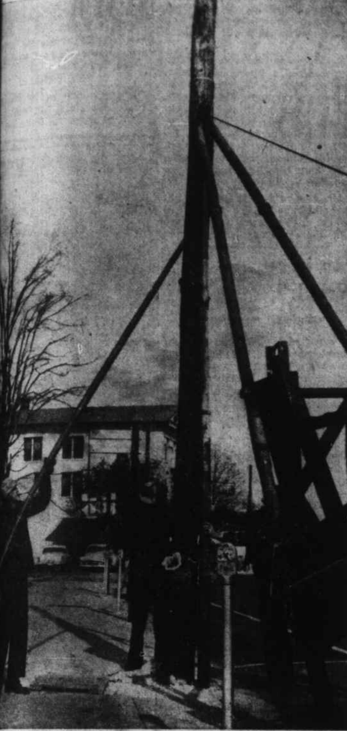
DOWN COME OLD WOODEN poles on Main Street, as they make way for the new steel poles of the modern whiteway. Town crews this week were pulling up all poles except those from which street lights were suspended. They will be removed as soon as new lights are installed. On the left, supervisor is Walter Sheaffey, in charge of the electrical department, while Bob Yarborough is guiding the pole as it comes out of the ground, and Fred Rogers can barely be seen behind the rigging of the truck. Earl Warren, not shown, was handling motor winch which pulled the pole. (Mountaineer Photo).
