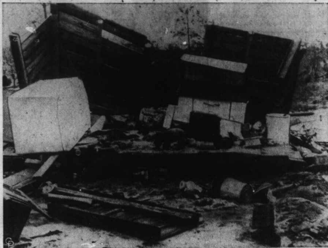
A PUPPY LOOKS AROUND for food in the wreckage of the Raymond Holley home, one of five demolished in Woodville, Fla., when several small tornadoes hit Gulf Coast towns without warning. The short-lived twisters, riding a storm front across the upper Gulf of Mexico, caused injury to at least 24 persons in both Florida and Louisiana. Seventeen were reported hurt in Woodville alone. (International Soundphoto)
