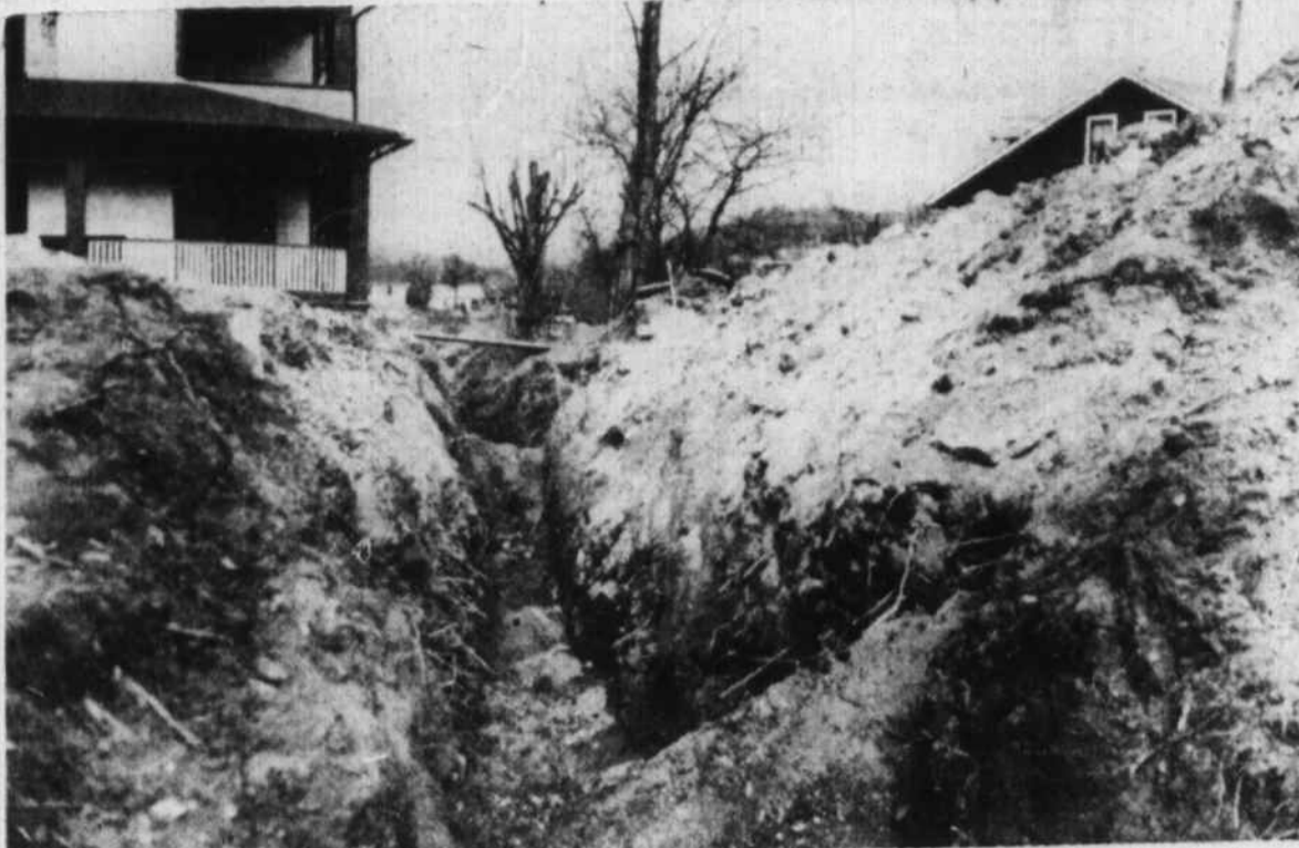
DEEP CUT was necessary across North Main Street for the new Shelton Branch sewer line. This photo shows the 14-foot cut across the street, which was filled up late Tuesday afternoon, and normal traffic resumed over the route. The line runs right near the home of Mr. and Mrs. W. L. Matney. (Mountaineer Photo).
