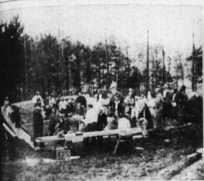
125 men built a home for J. A. Neff in one day. At 7:30 p.m. the structure was made. The home is near Mountain Sanitarium.
