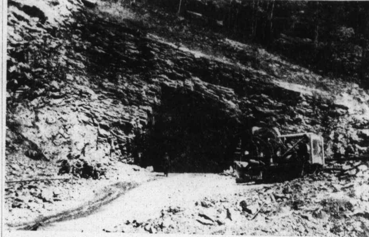
THIS TUNNEL being blasted through rock on the new Pigeon River Road will be one of the longest east of Maryville, at 1,035 feet. It is be- ing constructed at the end of the present 6 1/2- mile link by the Harrison Construction Co. of Pittsburgh, sub-contractor for the A. B. Burton Co. (See other pictures, Page 1, Section 2.) (Mountaineer Photo).
