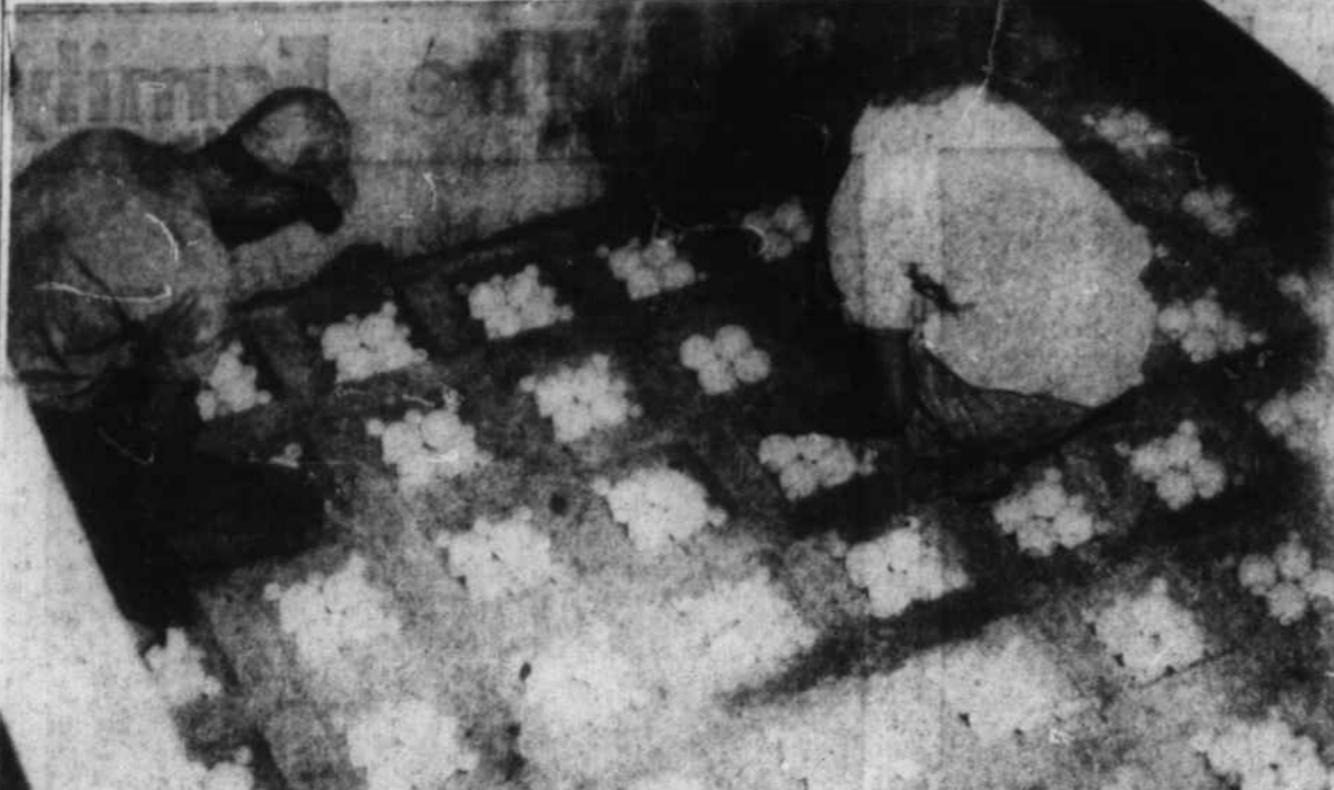
PORCELAIN BALLS of various sizes are placed on the bottom of filter beds in Waynesville's new filtration plant, which will start operation some time in August. Stone will be placed on these balls and on that a layer of sand to provide an effective filtration base. (Mountaineer Photo).
