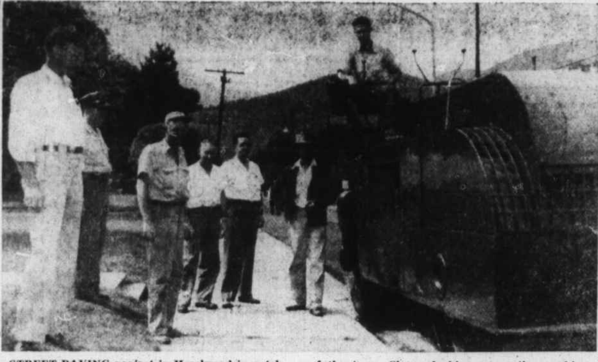
STREET PAVING project in Hazelwood is watched with interest by officials. The resurfacing of Main Street, with over 800 tons of asphalt, is a project of the state, but one worked up by the town officials, and the Finer Carolina Committee of the town. Shown looking on as the machine lays the asphalt include: Mayor Lawrence Davis, Aldermen John Blaylock, Howell Bryson, Chief Roy Stevens, Paul Bryson and A. P. Ledbetter. (Mountaineer Photo).
