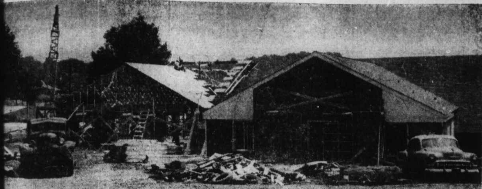
WORK IS PROGRESSING at a fast pace on the $80,000 Youth Center at Lake Junaluska. This picture, made Tuesday, shows a partial view of the front of the 4,800-square foot building on the lakeshore, near the swimming pool. The offering taken Sunday at "Junaluska Day" will be used for the building fund, which now amounts to about $50,000. (Mountaineer Photo).
