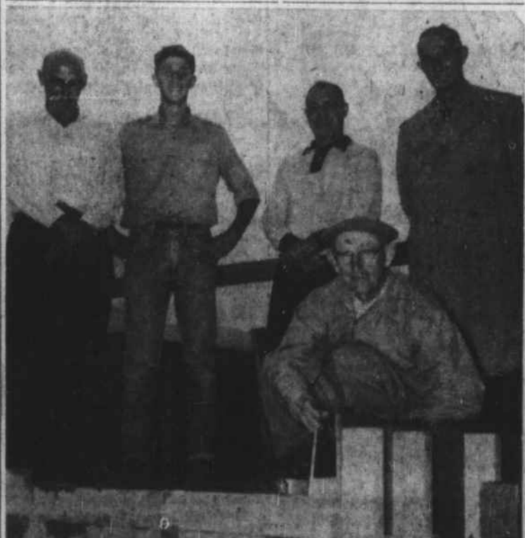
R. L. 'POP' PREVOST (kneeling), president of the Unagusta Furniture Co., sank two gold-plated anchor bolts in concrete Friday afternoon at the construction site of the company's new plant, where more than two-thirds of the steel has already been erected. Looking on here are Ralph Prevost, Sr., Ralph Prevost, Jr., Harry Crawford, and Whitener Prevost. (Mountaineer Photo).
