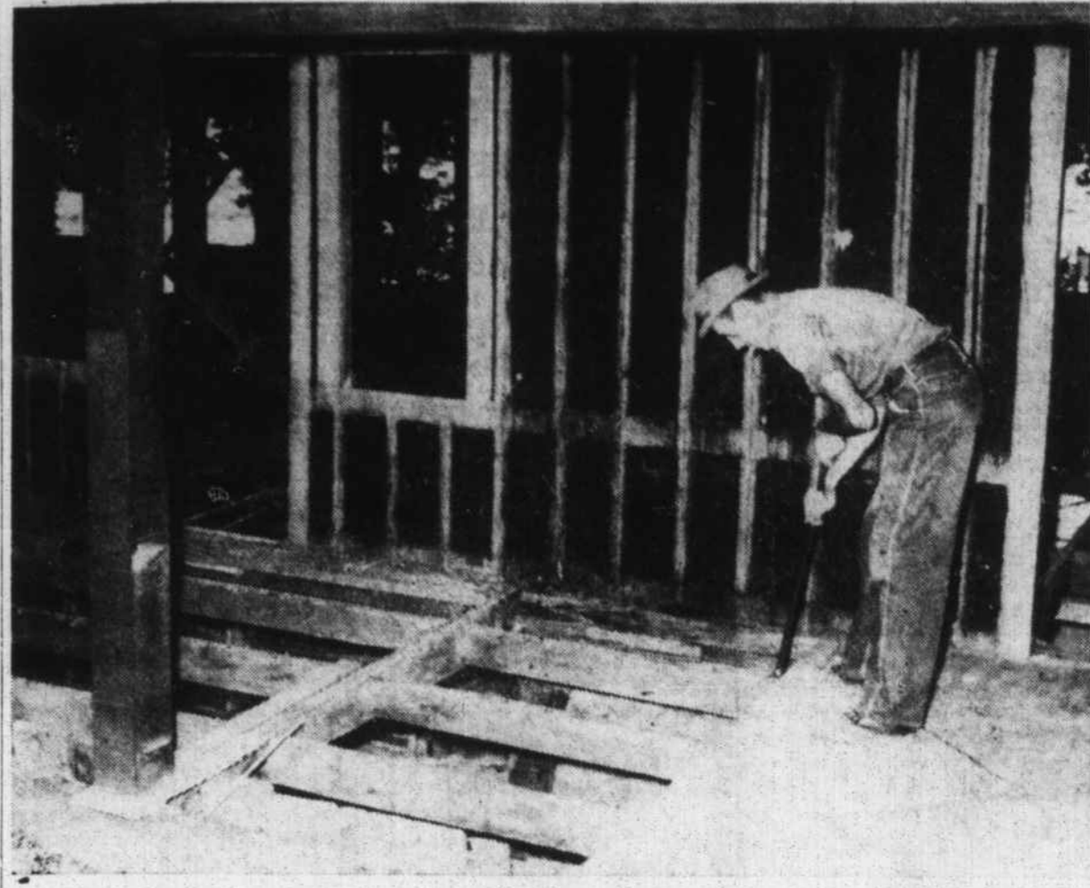
A WORKMAN tears down Mountain View Lodge, Lake Junaluska, to make way for a $250,000 structure which will have 128 beds. The new structure is just back of Shackford Hall, overlooking the back part of Lake Junaluska, and the Smokies in the distance. (Mountaineer Photo).
