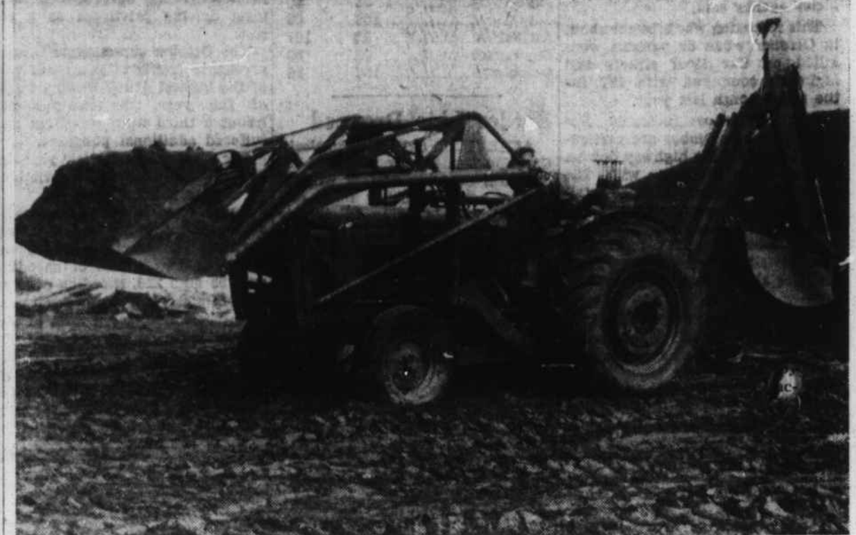
'JACK OF ALL TRADES' is this Diesel tractor with Sherman digger and Sherman loader which is now being used in local construction jobs. The machine handles all kinds of excavation, ditch digging, loading, septic tank work, driveway construction, backfilling, etc. The unit, seen here in operation at the site of W. L. Turner's new home on the Dellwood Road, was purchased by the John Norris Construction Co. of Waynesville from the Rogers Tractor Co. of Clyde.
