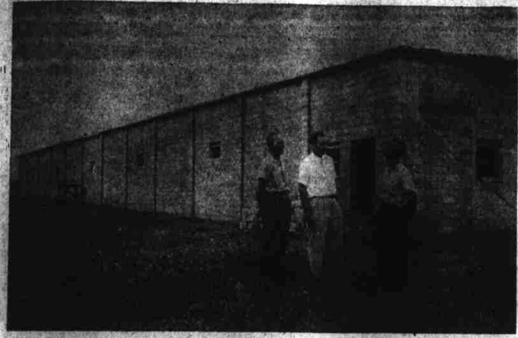
CABINET FACTORY - Shown above standing in front of Beulaville's New Cabinet Factory building, now under construction, talking over the progress and operations of the new plant are G. S. Muldrow Mayor of the Town of Beulaville, Leonard S. Cole, President of Southern Metals and Plastics Mfg. Co. of Norfolk, Va. and Woodrow Jackson of Beulaville, Manager of the New Beulaville Plant. The new industry is expected to begin operations in approximately two or three weeks. Plans are already being made for the expansion of the industry with the ultimate goal being an integrated manufacture of wood, metal and plastic products. (Photo by John Wells)
