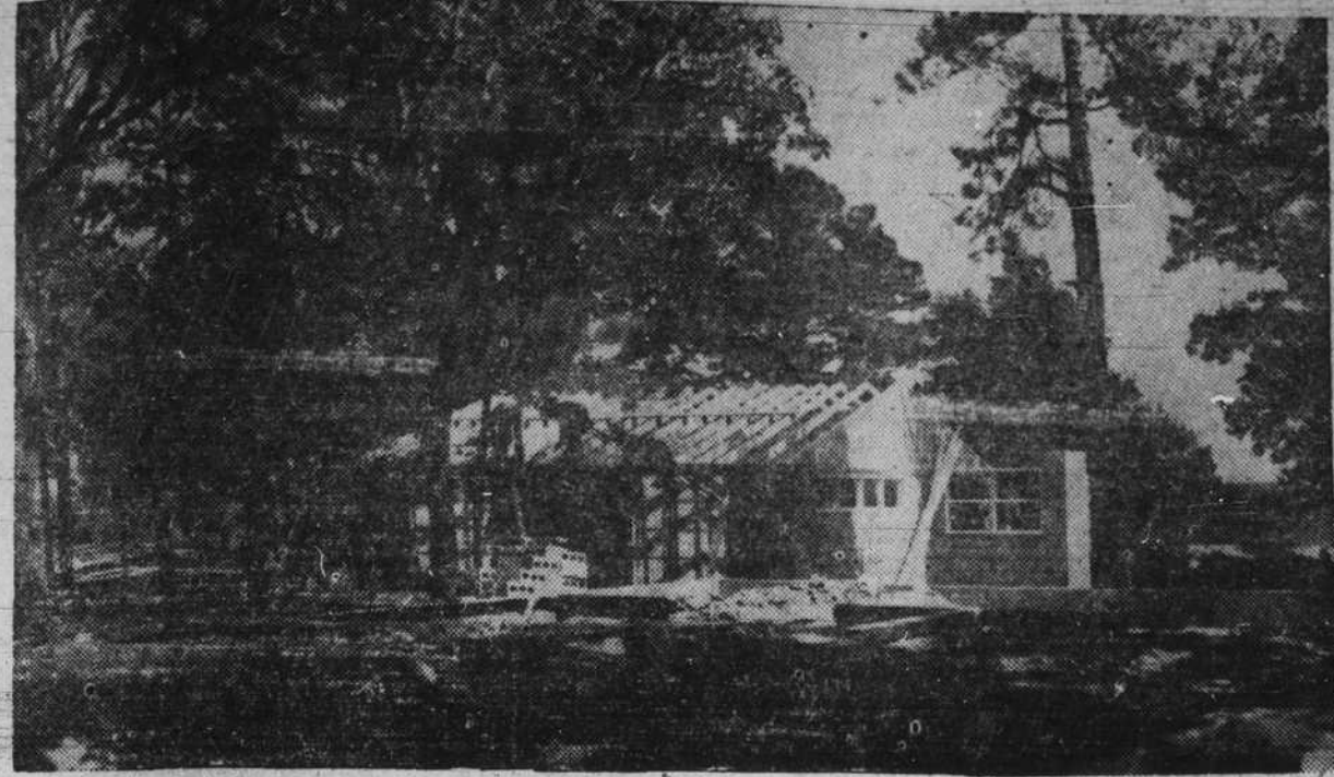
The photograph above shows the construction progress being made at Camp Don-lee, the Methodist Youth Camp of the North Carolina Conference. This camp is located on the north shore of the Neuse River, near Arapahoe, in Pamlico County. The camp site was donated to the Annual Conference by Mr. Don Lee and the camp is being constructed through the efforts and contributions of the 160,000 Methodist people of the North Carolina Conference.
