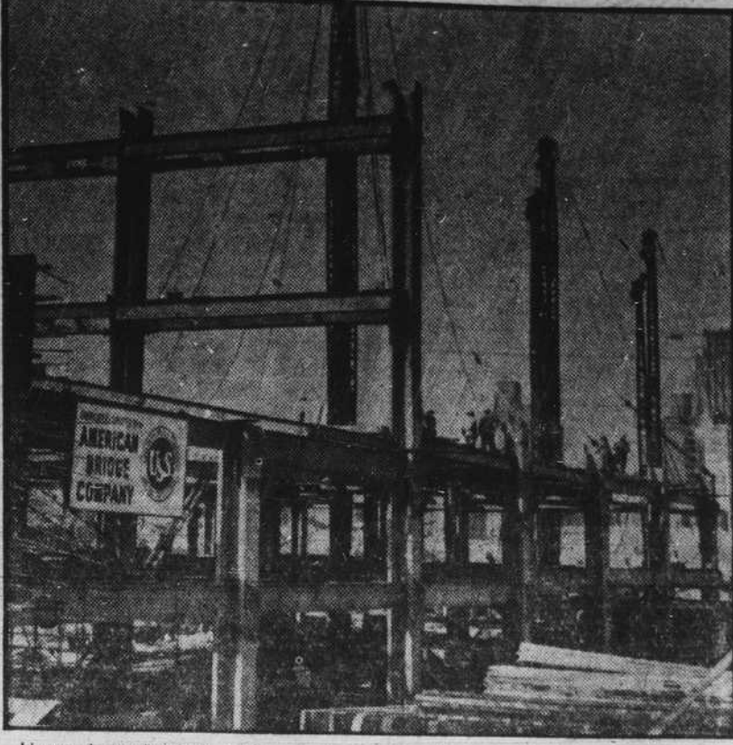
Huge derricks pull girders into position for the 39-story Secretariat Building, first and tallest building under construction at the new United Nations Headquarters site in New York. More than a thousand tons of steel have been erected on the project so far.
