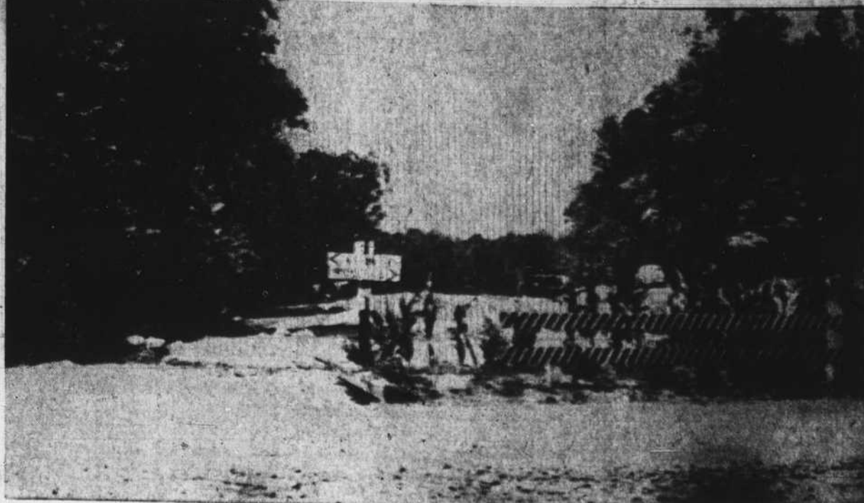
WORK IS WELL UNDERWAY on this new, shortened link of the Hillsboro highway. It will be two miles shorter than the present road via Airport Road to N.C. Highway 10 and into Hillsboro. The new road will leave the present highway just north of New Hope Church at the junction shown above and join it again at the Farmer's Exchange Livestock Market on N.C. Rt. 10 a mile east of Hillsboro. The State Highway Department is building the road with Orange County work crews.
